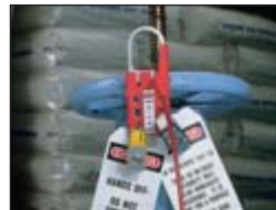
Lockout gate valves
